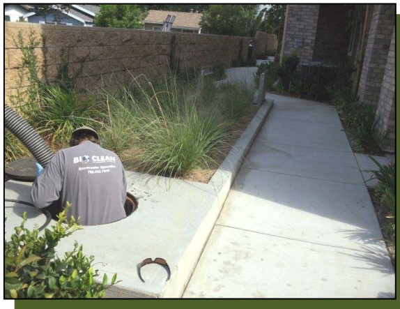
Vacuuming out of media filters.
