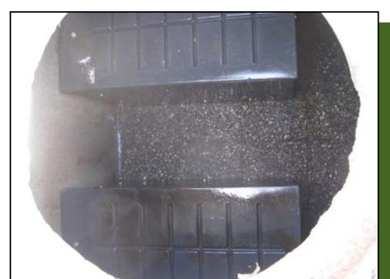
Fully cleaned separation chamber.
