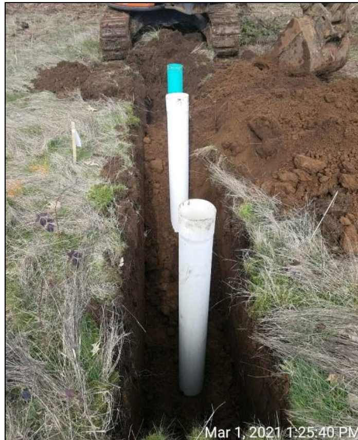
Photo 6: Setting the 3 standpipes in the test pit trench at one of the infiltration test locations.
