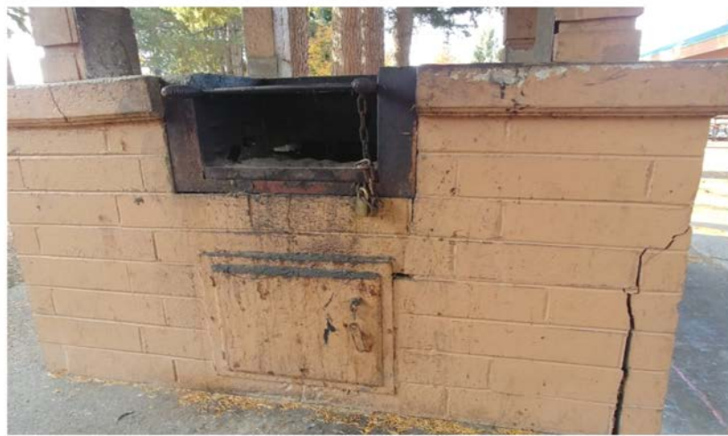
COMMUNITY PARK DETERIORATION
