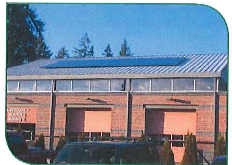
Solar panels installed at the Operations site on Herman Road.
