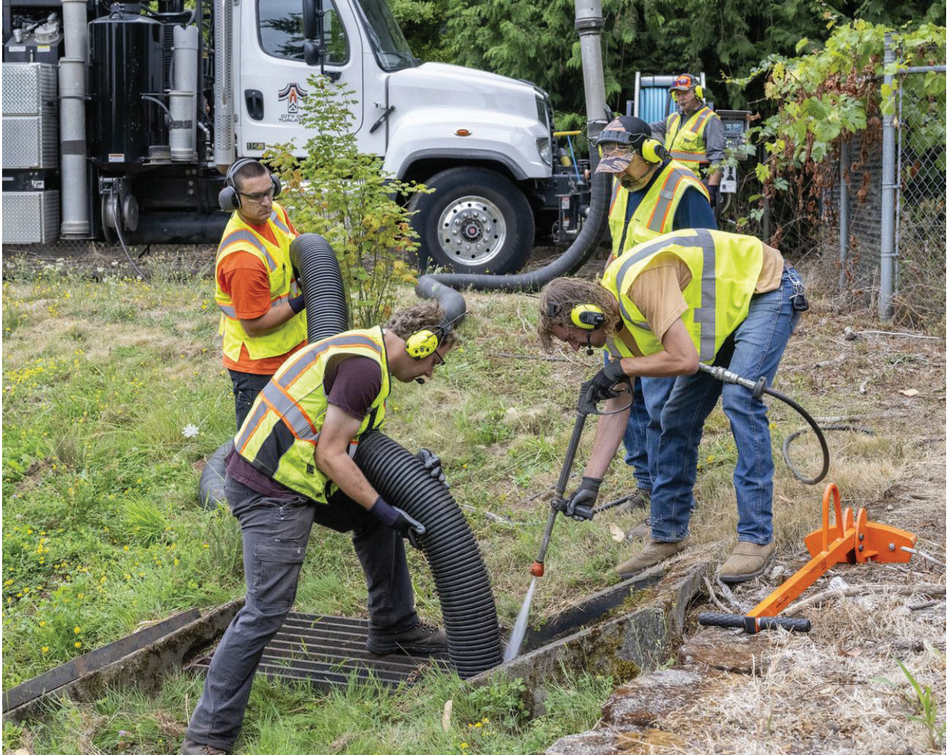
Public Works maintaining the sewer system
