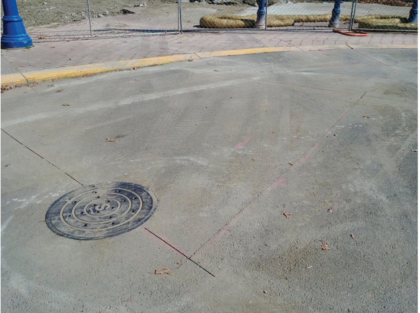
City storm drain
