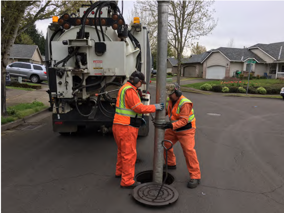
Cleaning Storm System
