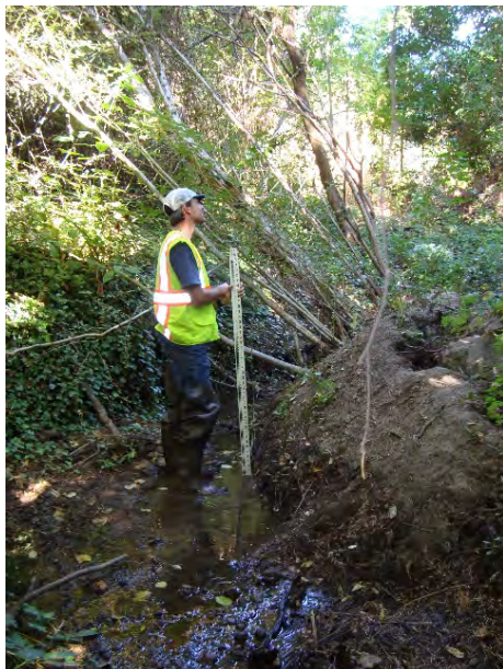
Photo 14. Left bank slump upstream of confluence.
