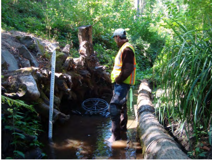
Photo 13. Restoration area showing cabled logs and root wads. Approximately 950 feet upstream of SW 105th Avenue.
