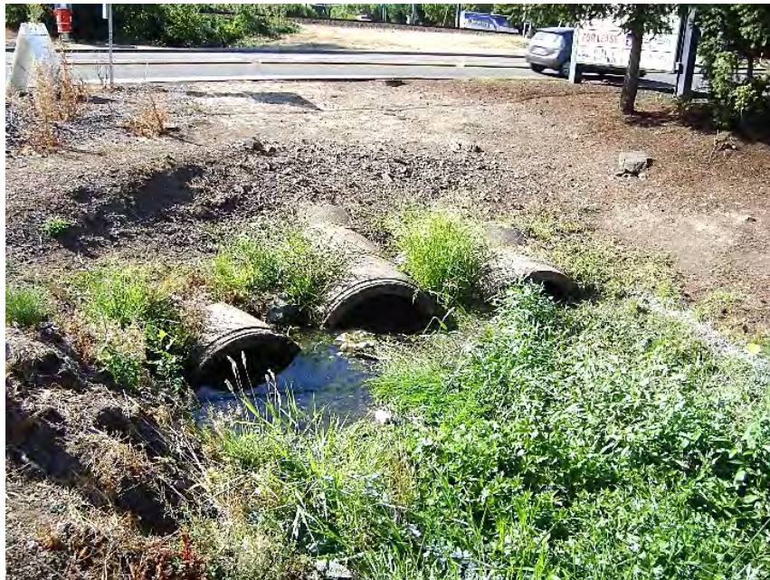
Site location: SW Boones Ferry Rd. Photo number: N3-10 Description: Culverts entering Nyberg Creek from SW Boones Ferry Rd.
