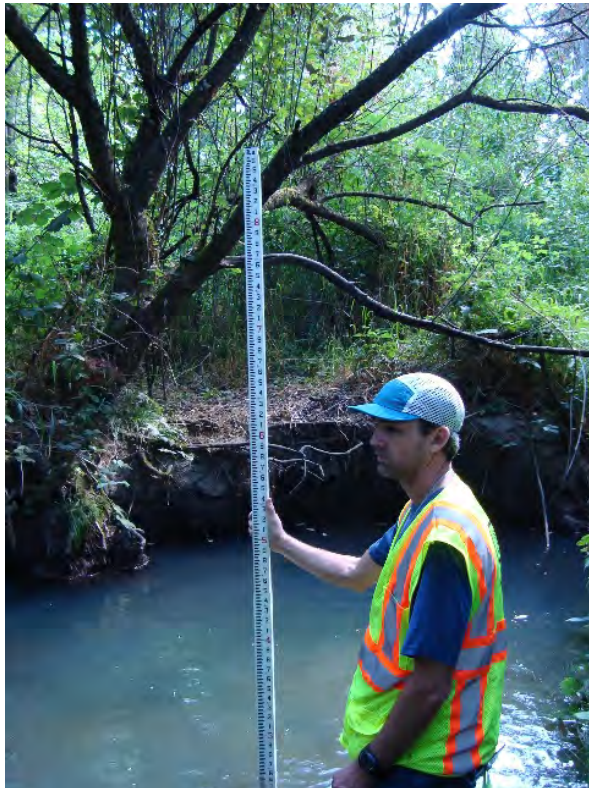
Site location: 600' upstream of SW Tualatin-Sherwood Road Photo number: H2-6 Description: Erosion on outside bend (right bank)
