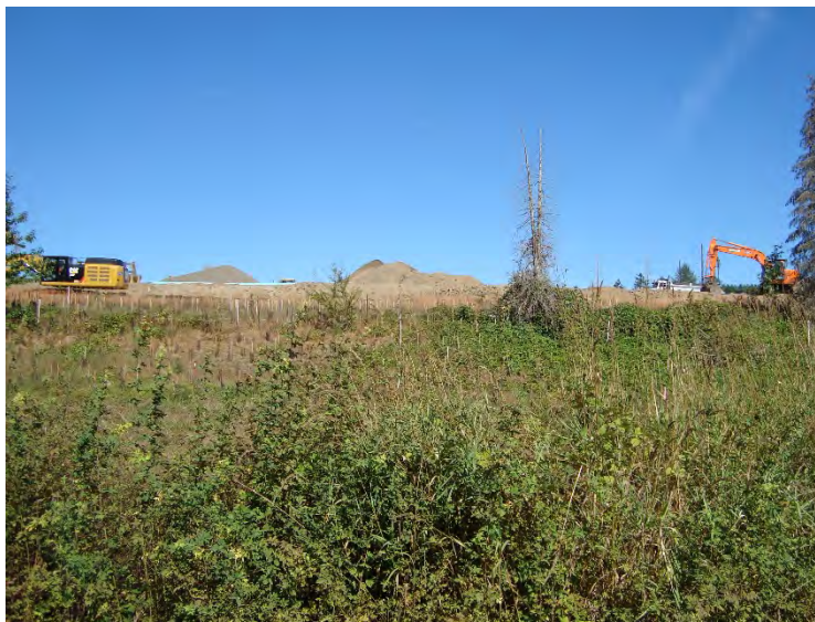
Site location: 1000' east of SW 65 th Ave. Photo number: S2-16 Description: Looking north at construction site across channel
