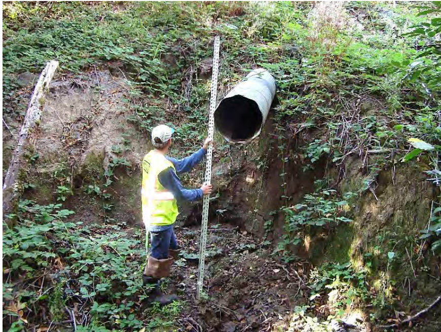
Site location: Downstream of SW Blake St. Photo number: S3-3 Description: Perched culvert- hillslope failure on left bank
