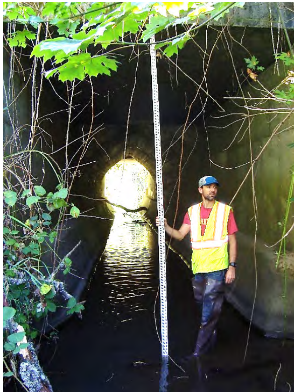
Site location: SW Borland Rd. culvert Photo number: S1-20 Description: Looking upstream (10 1/2' high, 10' wide)
