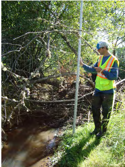
Site location: 100' east of SW 65 th Ave. Photo number: S2-18 Description: Debris jam looking downstream
