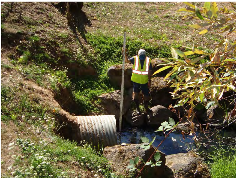
Site location: Culvert at SW Industrial Way Photo number: H2-14 Description: Looking down from right bank
