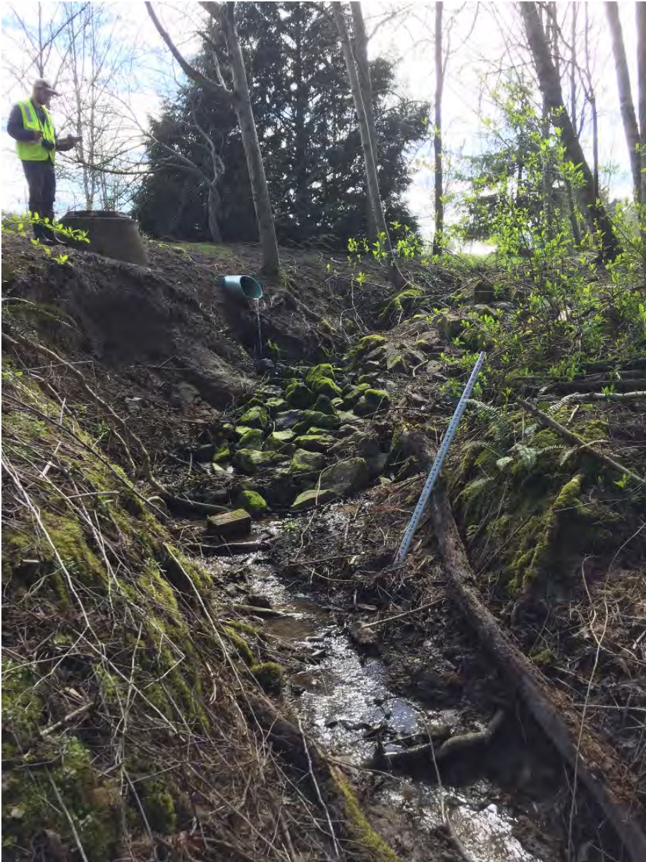
Image 2. Location 'N' outfall and channel erosion (photo provided by OTAK)
