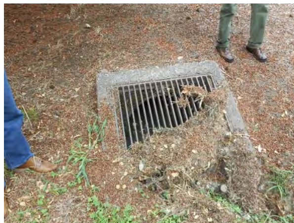
Image 2. Tree debris clogging the ditch inlet at the downstream end of the open channel
