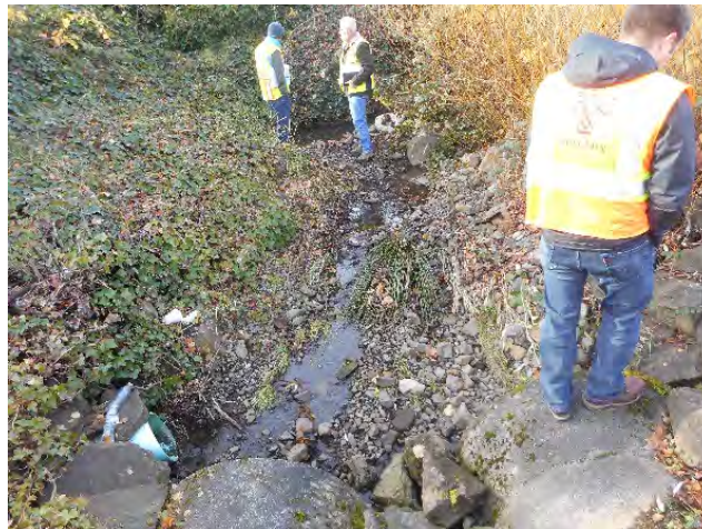
Image 2. Accumulated ballast and debris upstream of culverts across Boones Ferry Road
