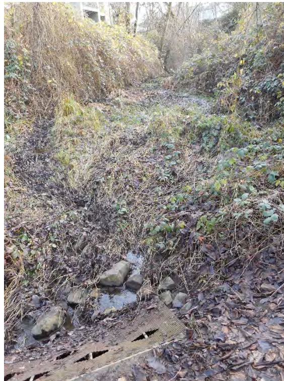
Image 1. Grated inlet and open channel near Mohawk Apartments
