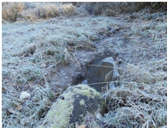
Image 2. Sediment deposition near outfall of stormwater system
