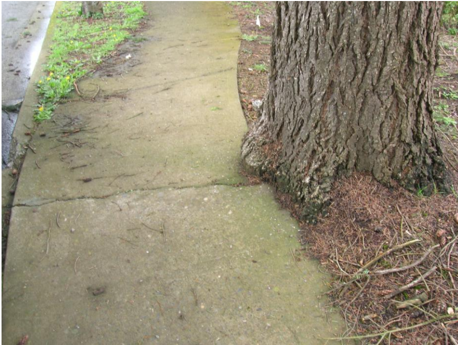
Douglas Fir #1266 – Already Heaving Existing Sidewalk
