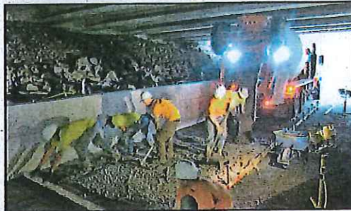
Brown Contracting employees place concrete for path under I-5. Fencing, railing, and daytime lighting will be installed before the trail opens in the Winter of 2015/2016.
