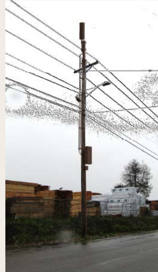
Utility pole with antenna
