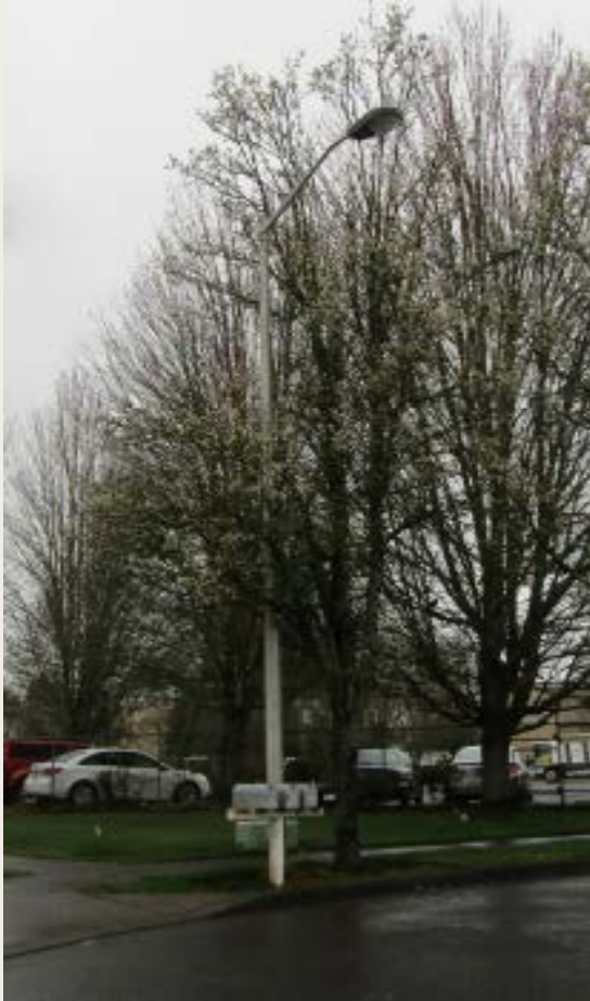
Existing street light
