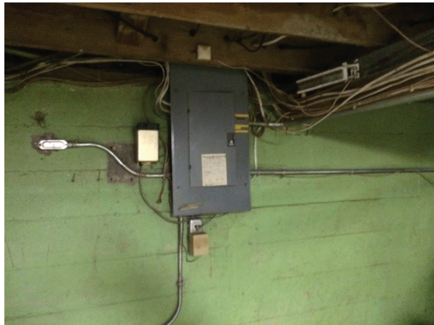
Figure D50.6 Electrical panel at Basement
