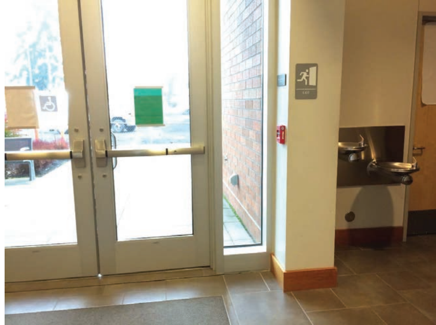
Figure D60.3 Typical fire alarm pull at building entrance/ egress doors
