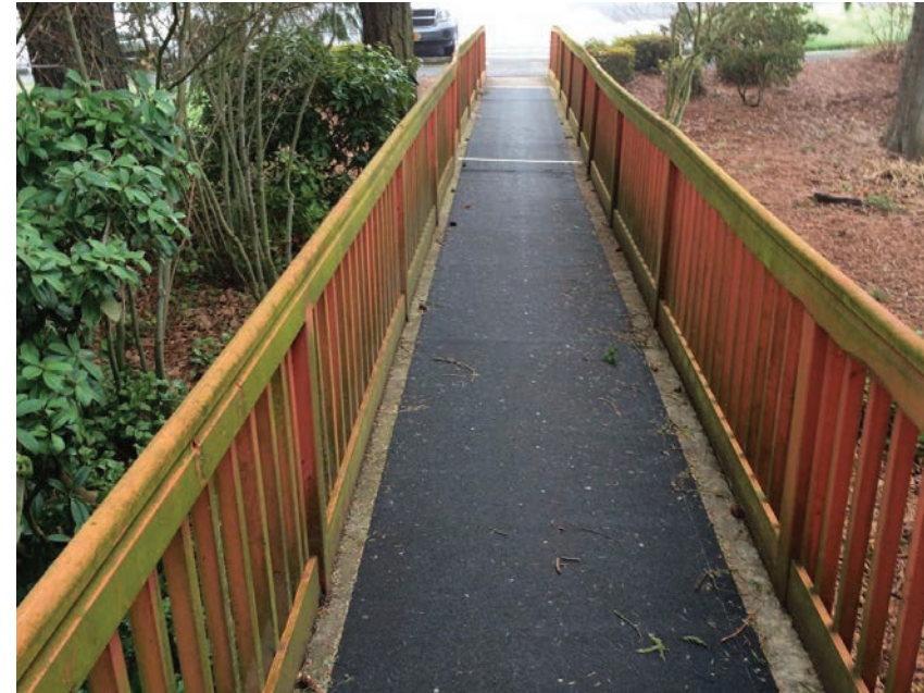
Figure C10.4A Main entry is accessible via ramp from parking area (south)
