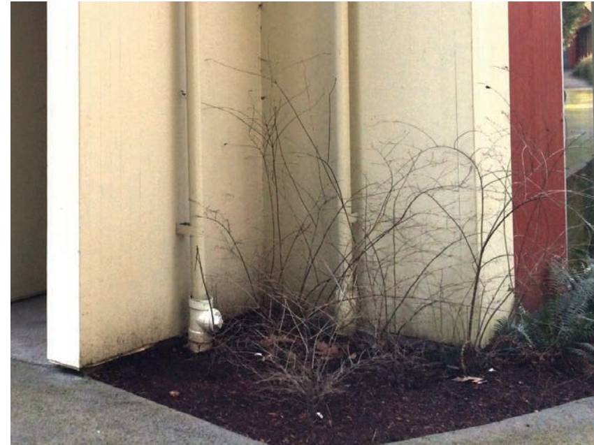
Figure G20.8 Soil and topping in contact with siding at rear (northeast corner)
