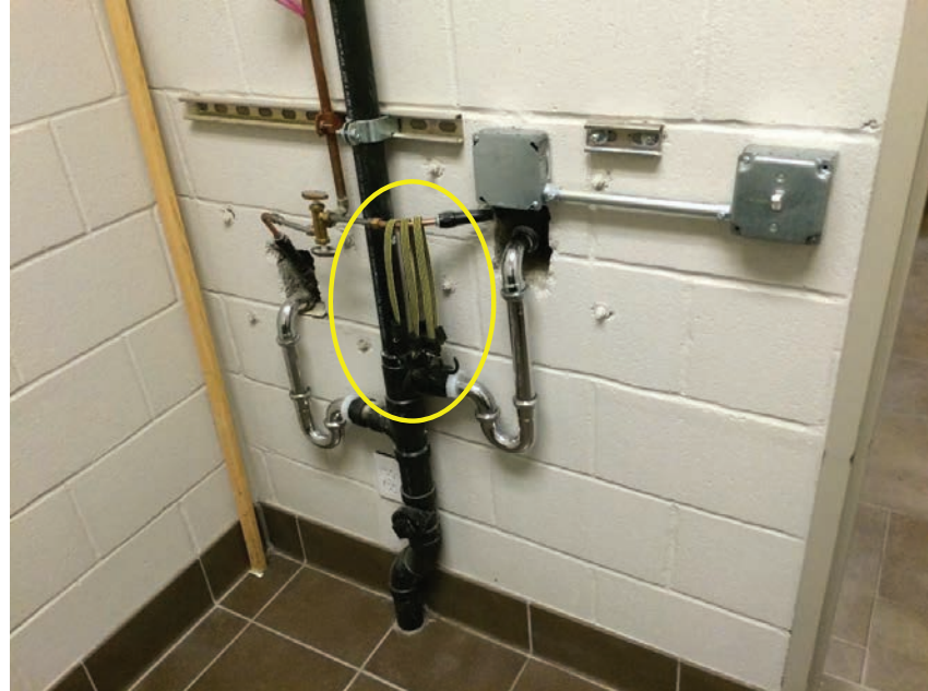
Figure D20.1/8 Copper water supply and PVC sanitary lines; note straps hung from plumbing
