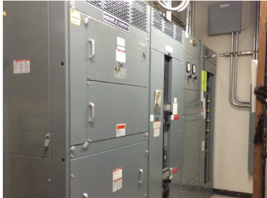
Figure D50.11 Main distribution equipment serves both portions of the facility from Electrical room
