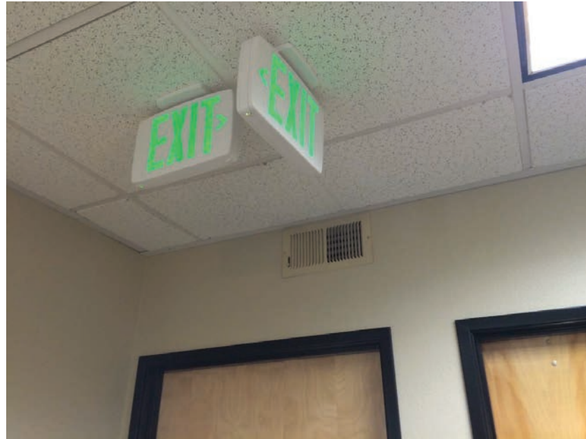
Figure D50.27 Typical exit signage at common area corridor
