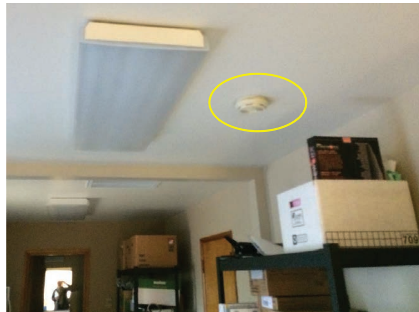
Figure D60.2 - Local, battery-operated residential type smoke detectors
