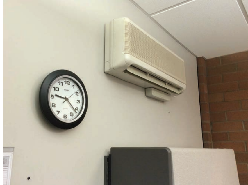
Figure D30.4B Remote split systems provided at south-facing offices in original portion of building
