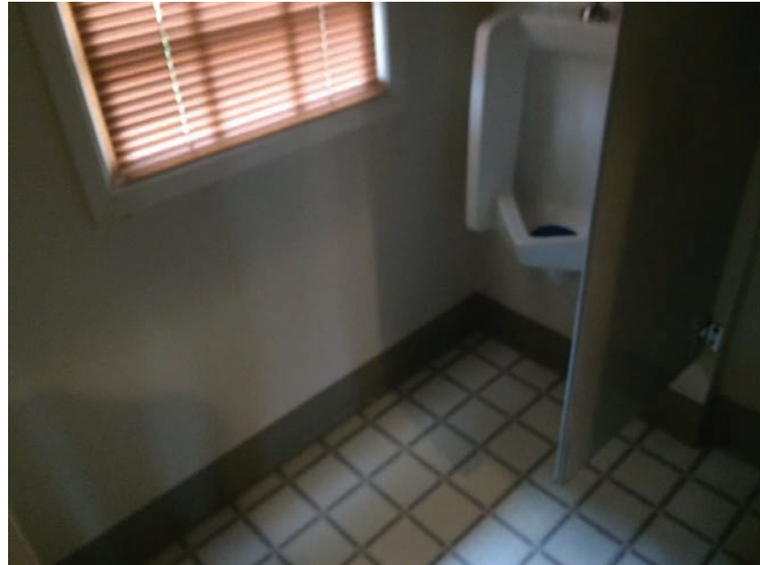
Figure C10.4C Restroom conversion from residential to commercial is not accessible
