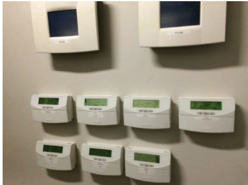
Figure D30.8 HVAC controls at Library
