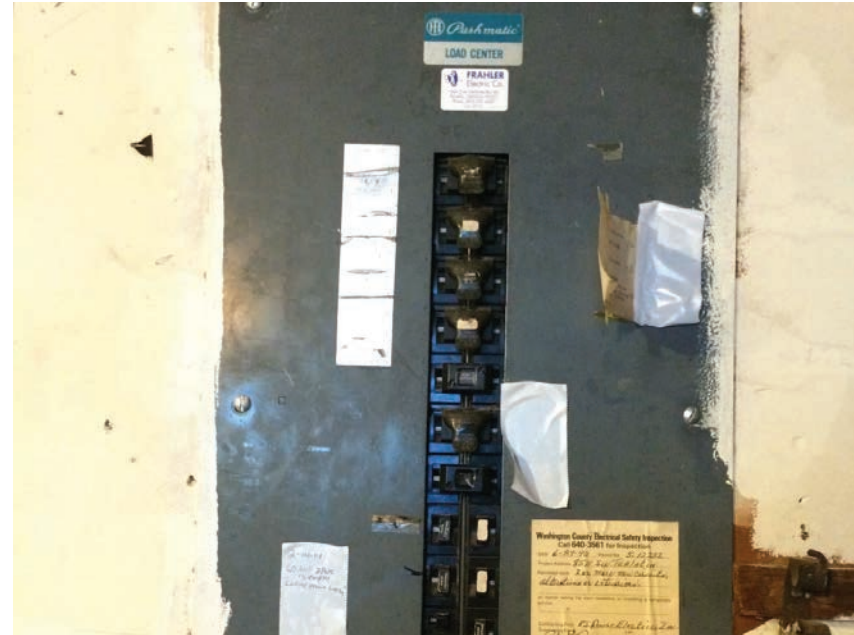
Figure D50.6 Original electrical panel with push button-type circuit breakers
