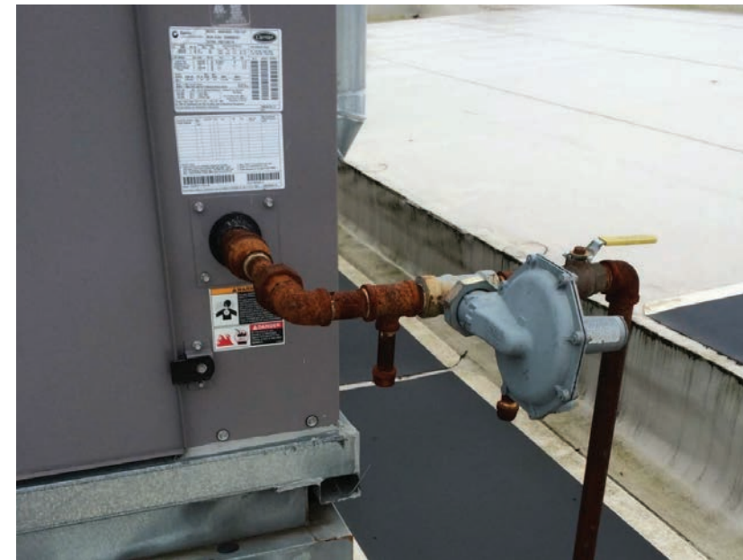
Figure D30.4A Rooftop mechanical units are gas-fired; typical gas line is unpainted pipe, corroded
