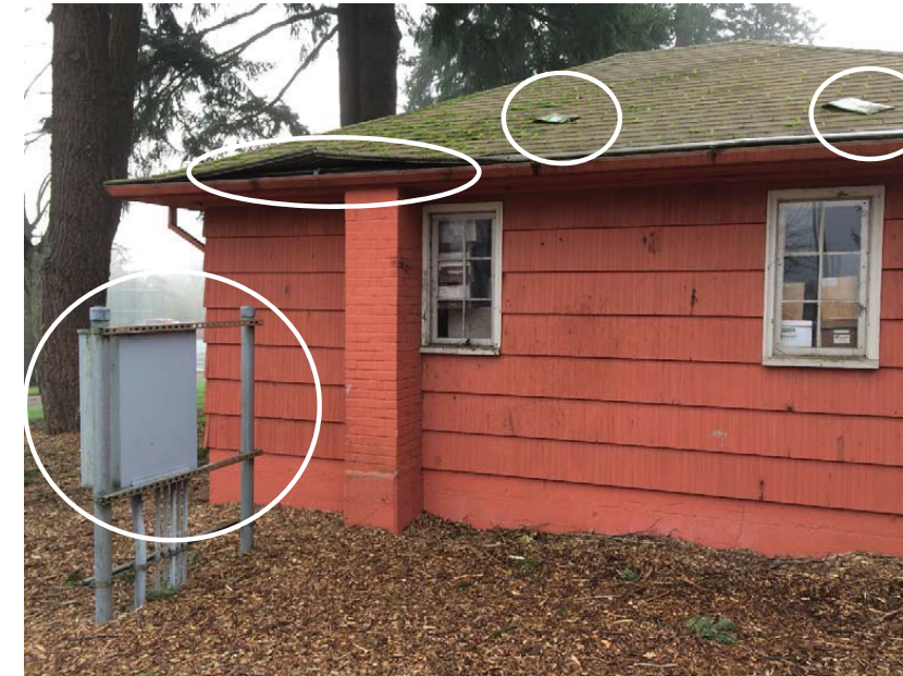
Figure B30.2 Damage at eave edge of Garage roof; Staff indicated that following the inspection, the observed damage at the Garage roof had been repaired; roof access may be possible by adjacent electrical equipment; abandoned skateboard decks on Garage roof
