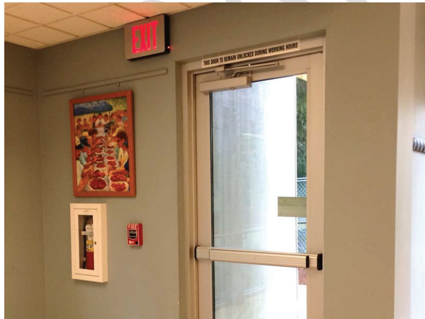
Figure D40.12 Fire extinguisher and fire alarm pull station adjacent to egress door
