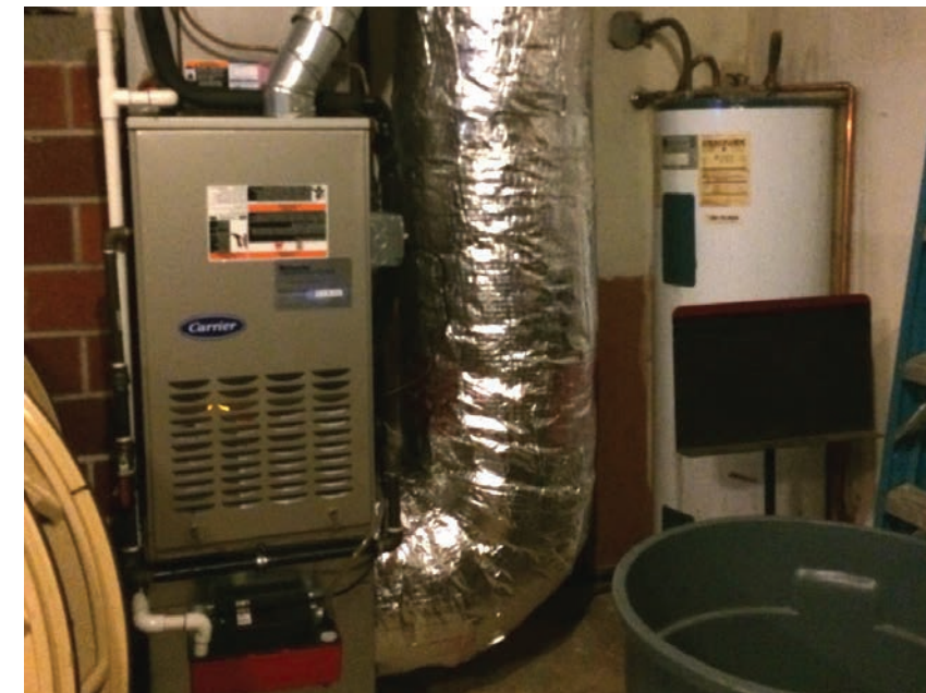
Figure D30.6 Air handler configuration; access compromised by storage
