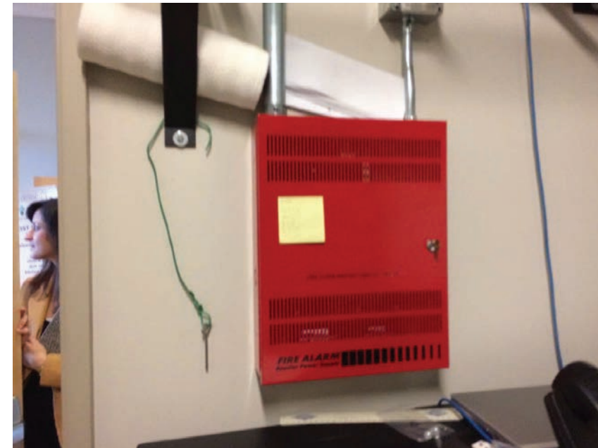
Figure D60.1 Main fire alarm panel in IDF room adjacent to Library Lobby
