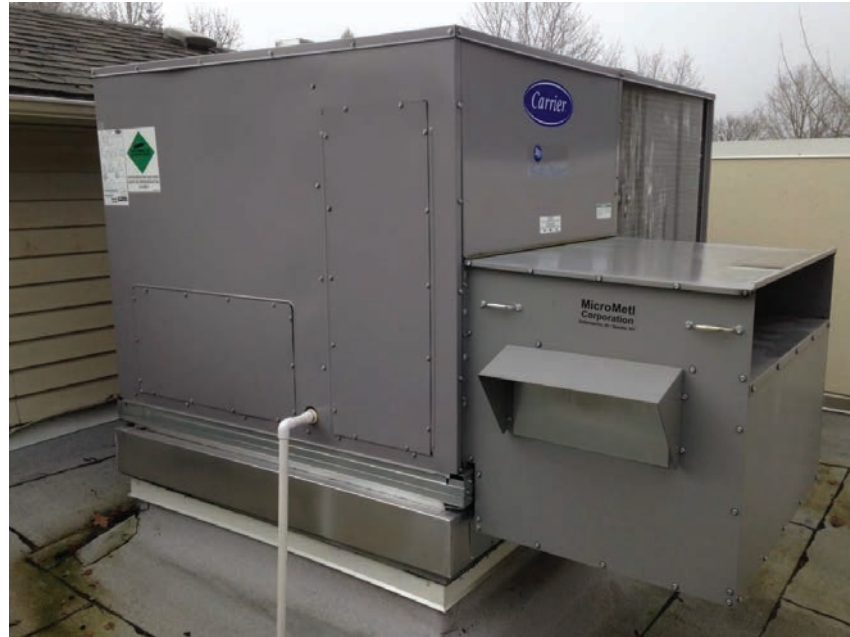
Figure D30.6 Staff photo of air handler configuration and access above Activity Room space
