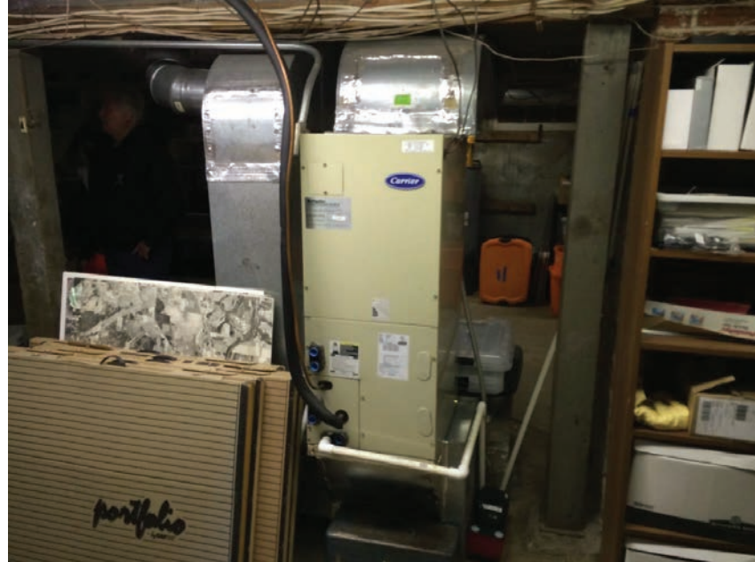
Figure D30.6 Air handler configuration and access at Basement
