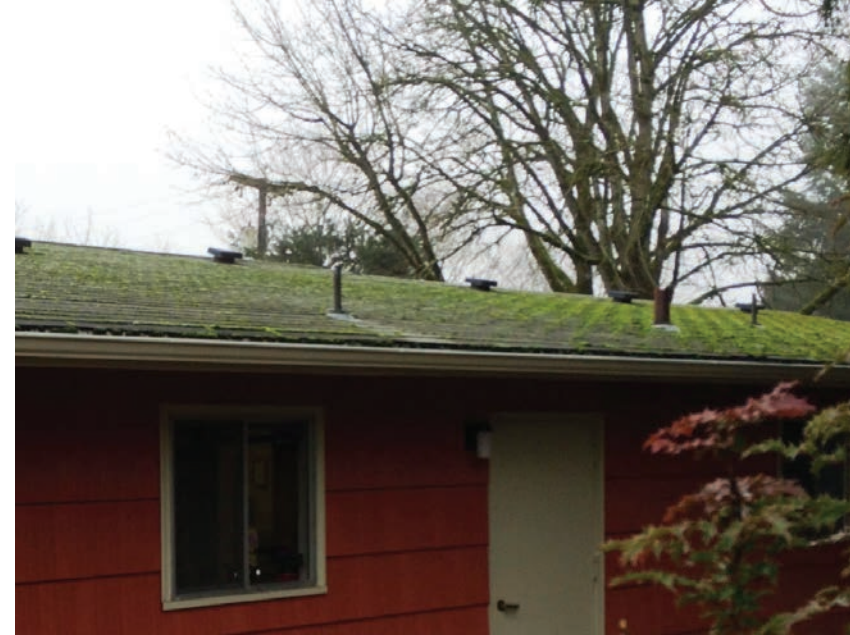
Figure B30.1 Moss at north roof
