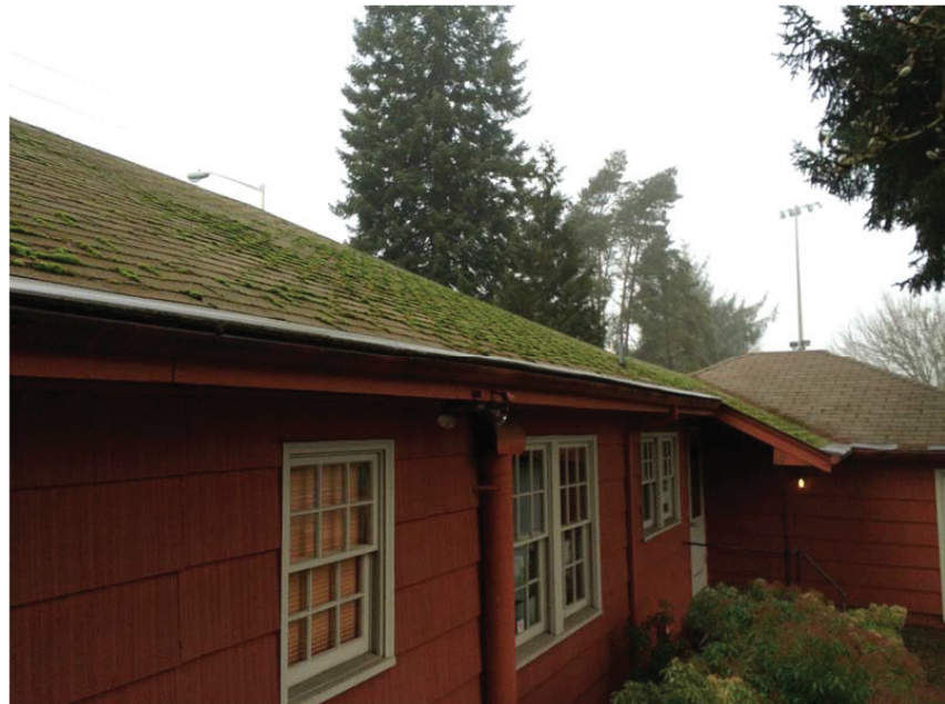
Figure B30.1 Moss at east side of roof
