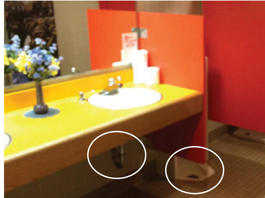
Figure C10.4 Sink and urinal are not accessible (Men's Room observed)
