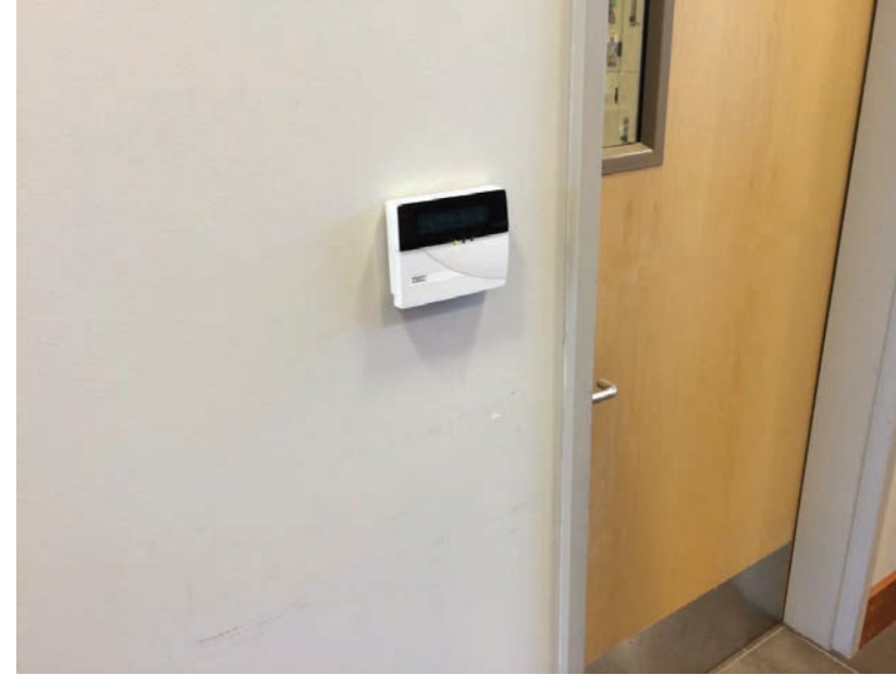
Figure G20.3B Security alarm remote keypad at City offices Lobby adjacent to door from City Offices Lobby to Library Work Room
