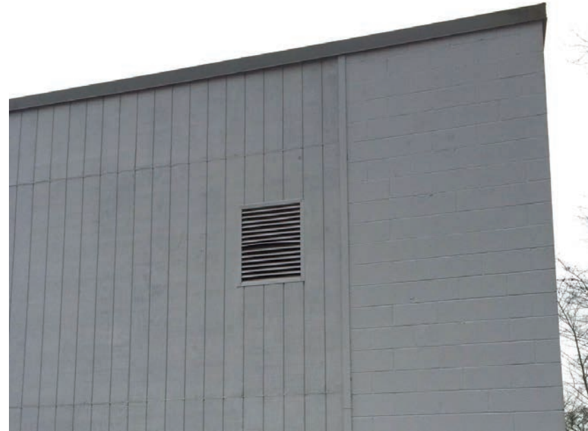
Figure B30.1C Louver at north is disused, staff noted that capped at interior
