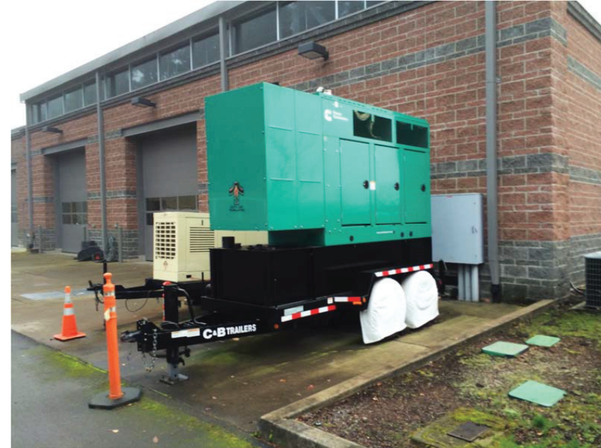
Figure D50.21 Trailer-mounted engine-generator set with base tank
