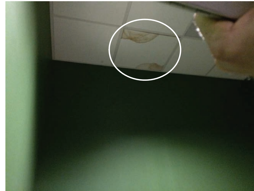
Figure C30.2 Evidence of leak visible in acoustic ceiling tile in Library
