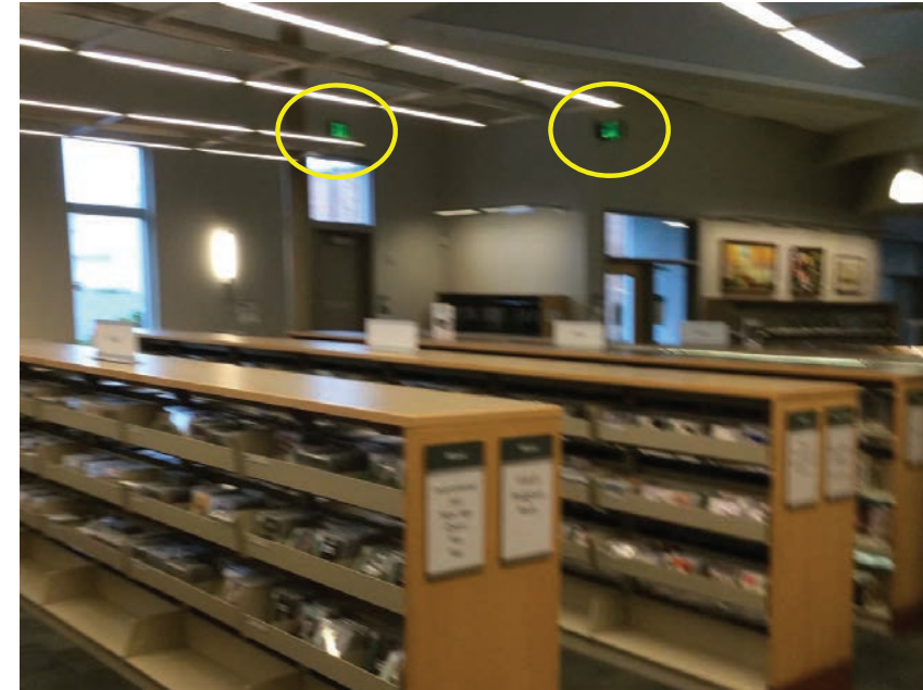
Figure D50.27 Typical exit signage is appropriately placed
