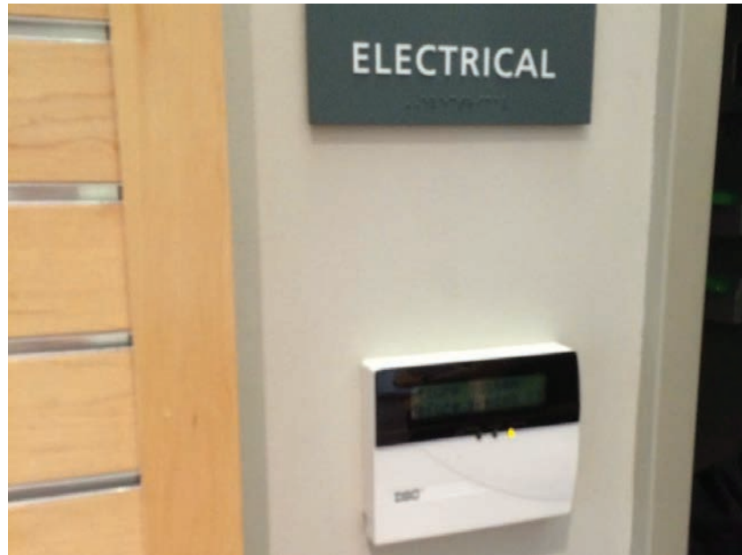
Figure G20.3A Security alarm remote keypad at Library Lobby adjacent to Electrical Room door
