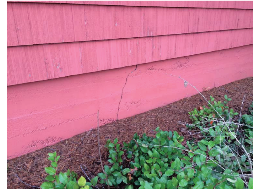
Figure A10.1 Minor cracking observed at basement walls (this location at south side)
