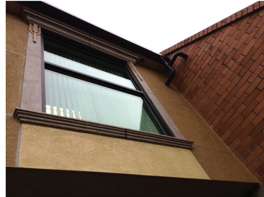
Figure B30.1 Metal roof edge, flashings and gutters appear to be in good condition
