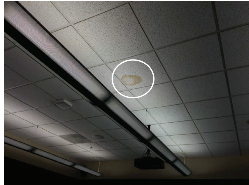
Figure C30.2 Evidence of past leak visible in acoustic ceiling tile; Staff noted that leak was repaired
