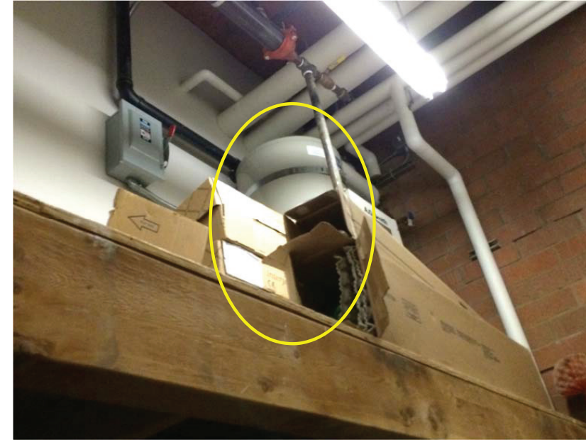
Figure D20.7 Water heater on wooden platform in Janitor room; appears to be seismically restrained; maintenance compromised by storage and limited access
