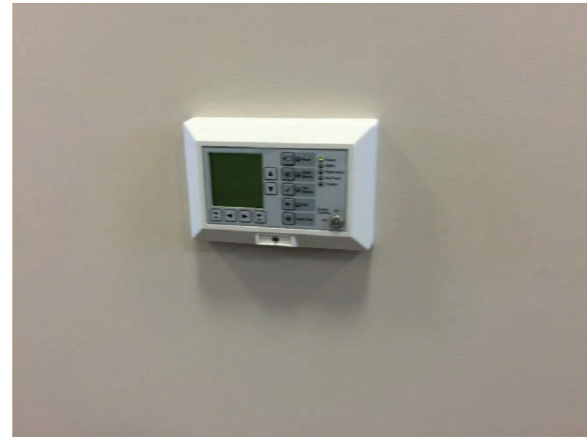
Figure D40.12 Fire alarm remote annunciator at Lobby
