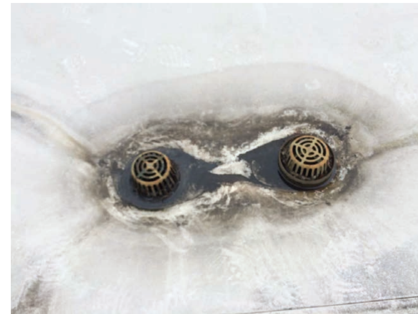
Figure B30.2 Typical roof drain and overflow drain conditions
