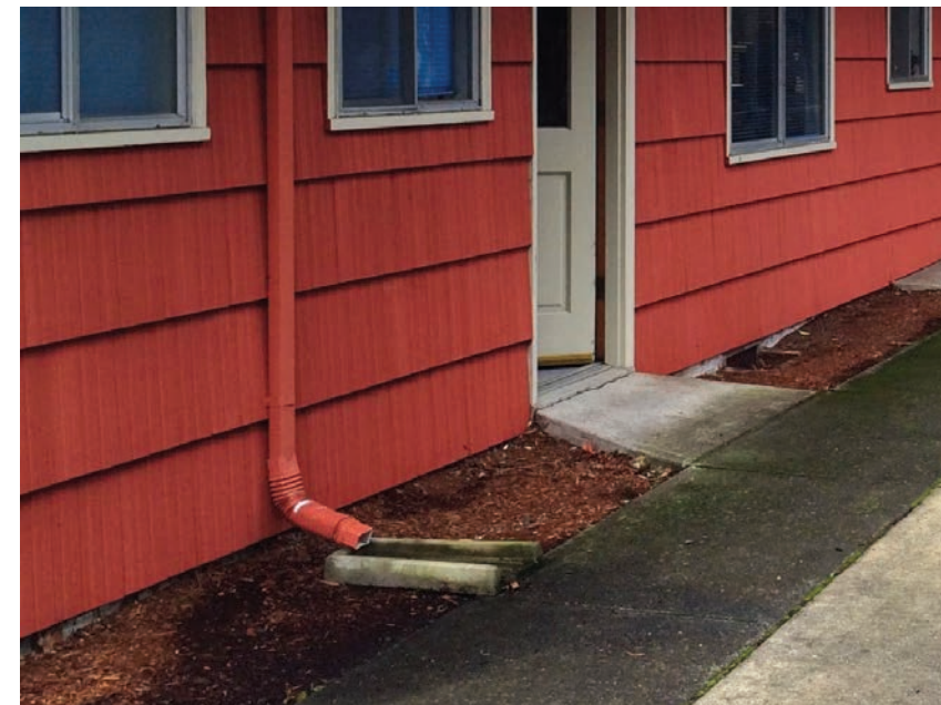
Figure G20.8 Soil and topping in contact with siding at rear (north)
