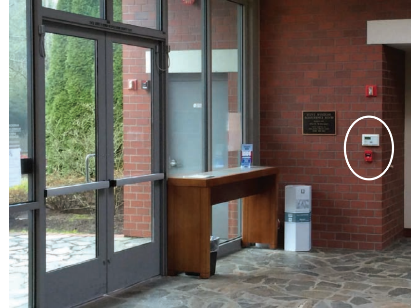
Figure D40.12 Fire alarm pull station and system panel adjacent to entry door
