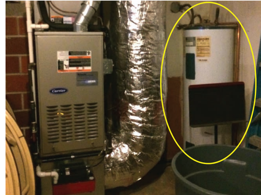
Figure E10.1 Water heater is not restrained for seismic forces
