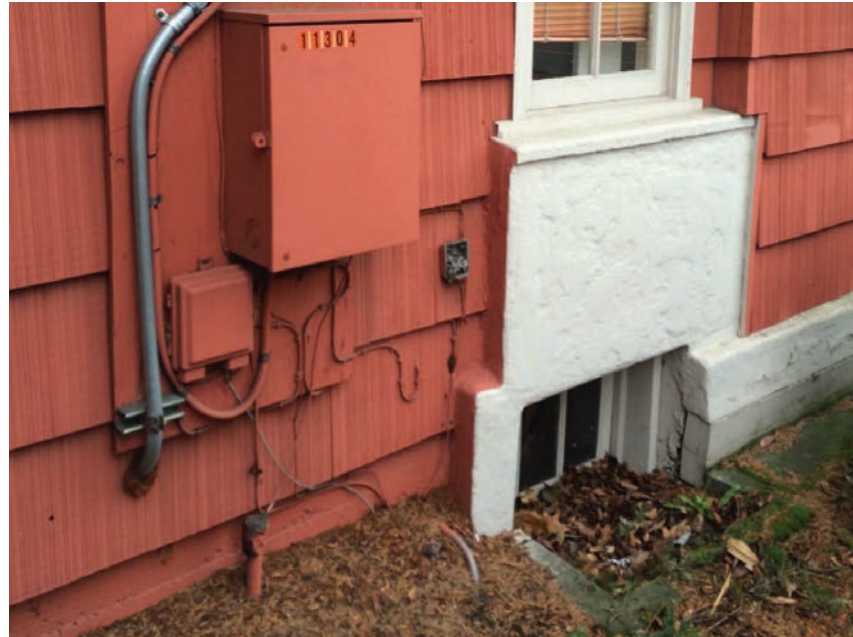
Figure B20.3 Window wells at Basement have collected leaves and debris at rear (east)
