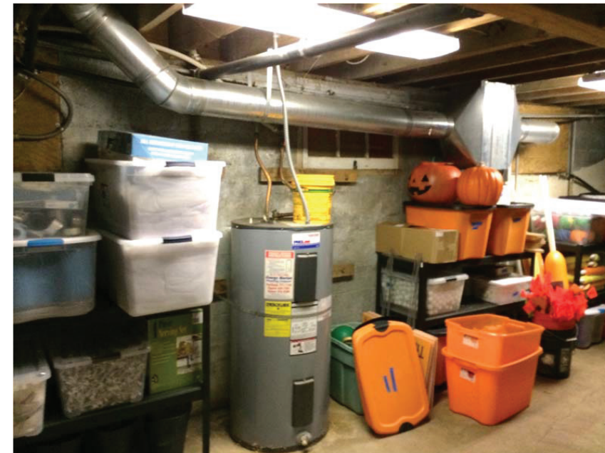
Figure E10.1 Water heater is restrained for seismic forces; clearances could be compromised
