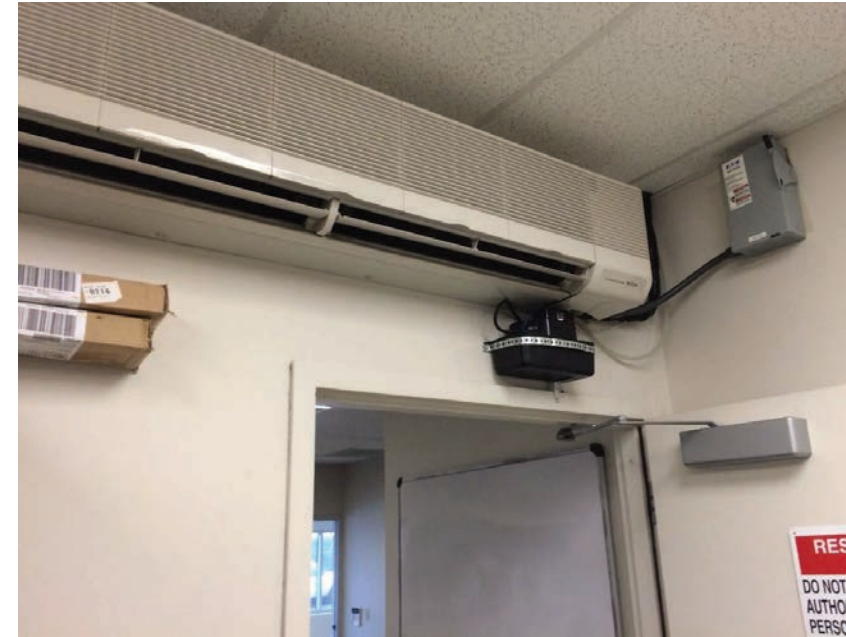
Figure D30.7 Split system HVAC at Server room; condensate pumped to disposal thru plenum
