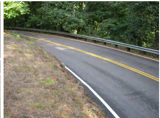
SW Blake Street and SW 105 th Avenue lack of shoulder
