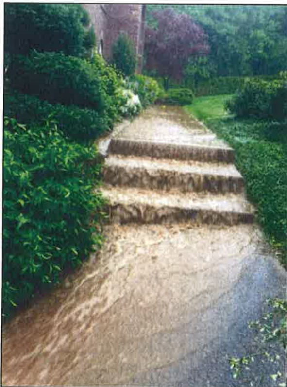
Photo A6. The front walkway steps drain into the lower driveway and garage area.
