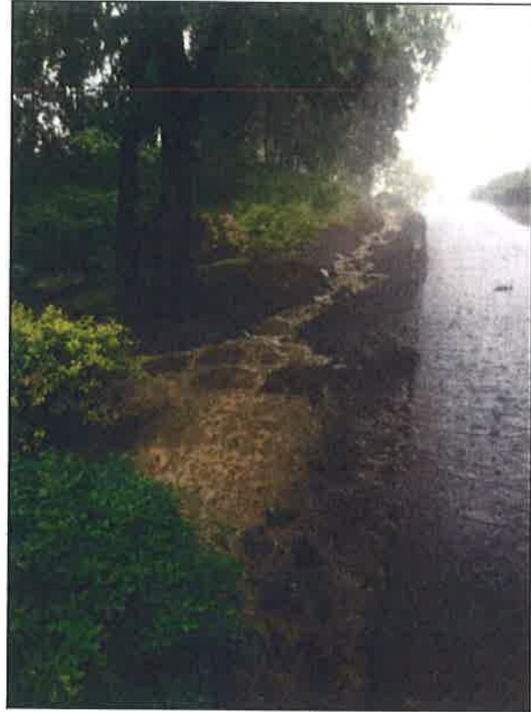
Photo A3. The junction for the channel and driveway pipe are overwhelmed and flood waters drain into the front yard toward the house.
