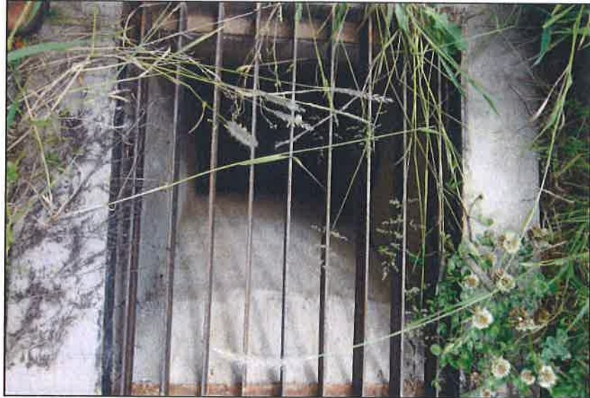
Photo B1. New Stormwater Inlet #1 (North).
